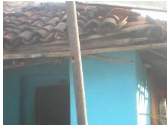
The iron pole has been pierced.
