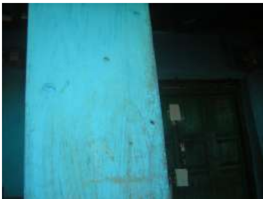
The holes caused by the splinters of the explosive device.
